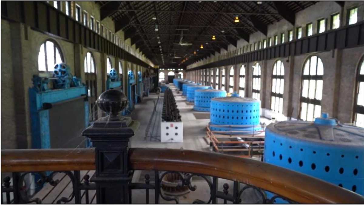
AC power station
